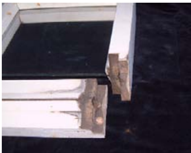
Figure 4.4: Slight decay in the rebate of a boron-treated E. obliqua window frame.
