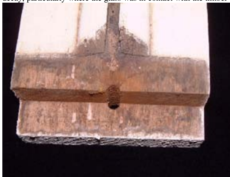
Figure 4.5: Decay in a window frame made from E. regnans treated with the current commercial LOSP formulation.
