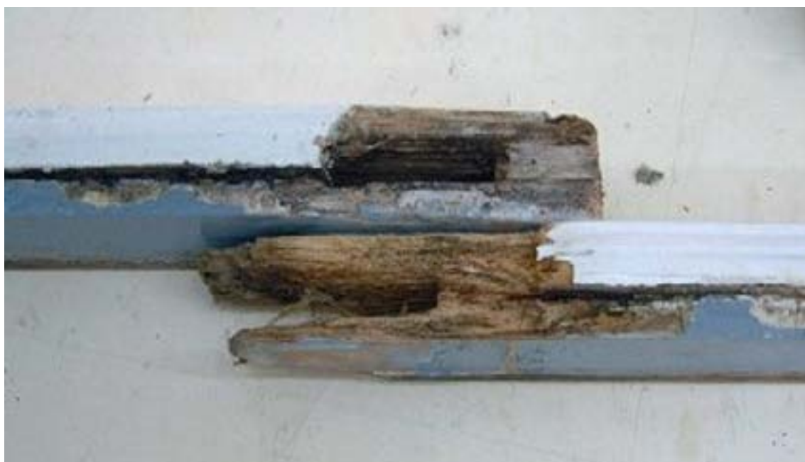
Figure 1.3: White rot in bottom joint of dismantled 50 year-old eucalypt window.
